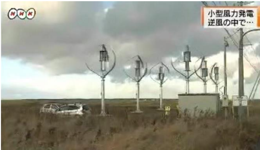
Small scale power plant, Nemuro, Japan
