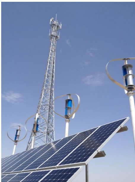
China Mobile telecommunication station, Xinjiang, China
