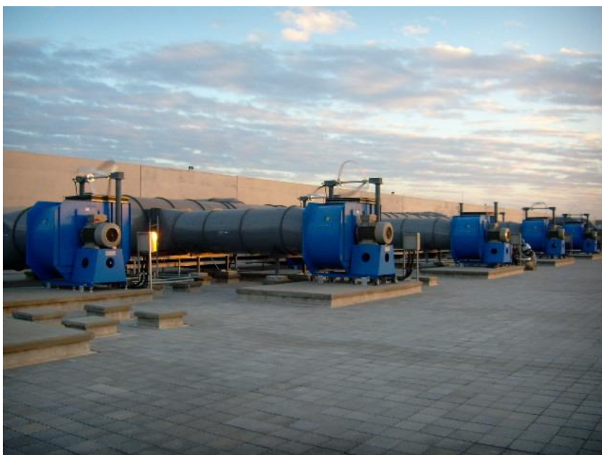
Energy recovery system at AU Optronics, Taichung, Taiwan
